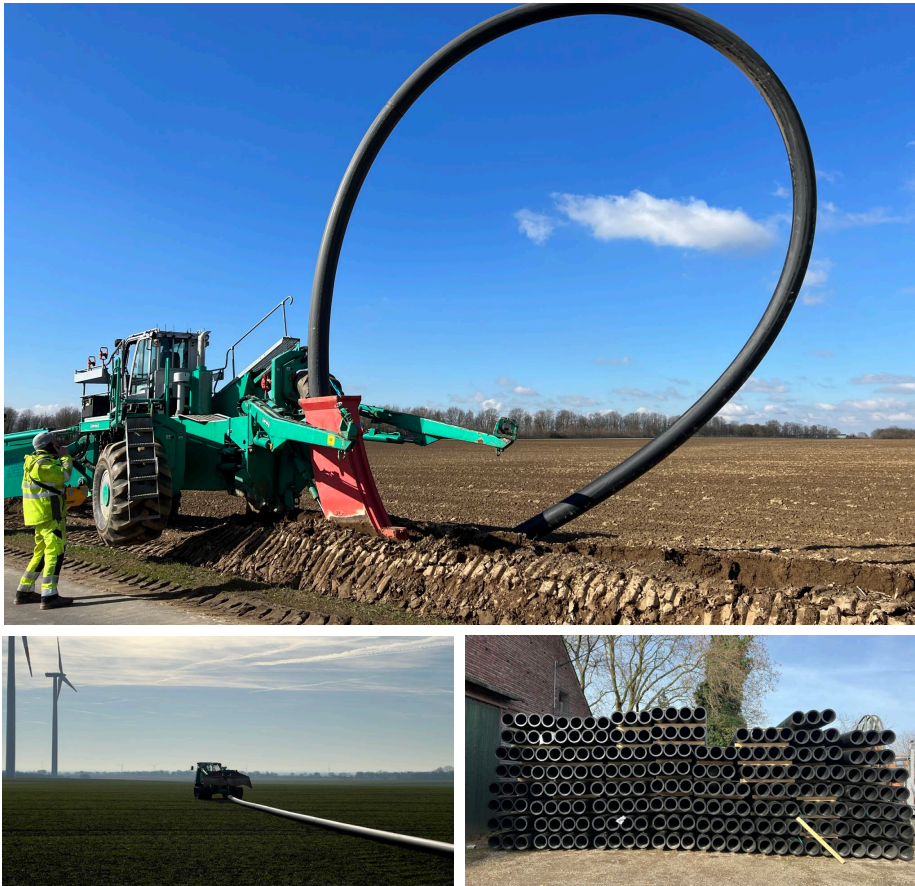
Top: installation of SIMONA pressure pipes by means of the ploughing method; bottom left: laying out the pipes; bottom right: SIMONA PE 100-RC Line pressure pipes
